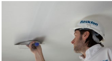
4. Once the first coat dries*, apply a second coat of filler to all joints and fasteners to guarantee good overall evenness
